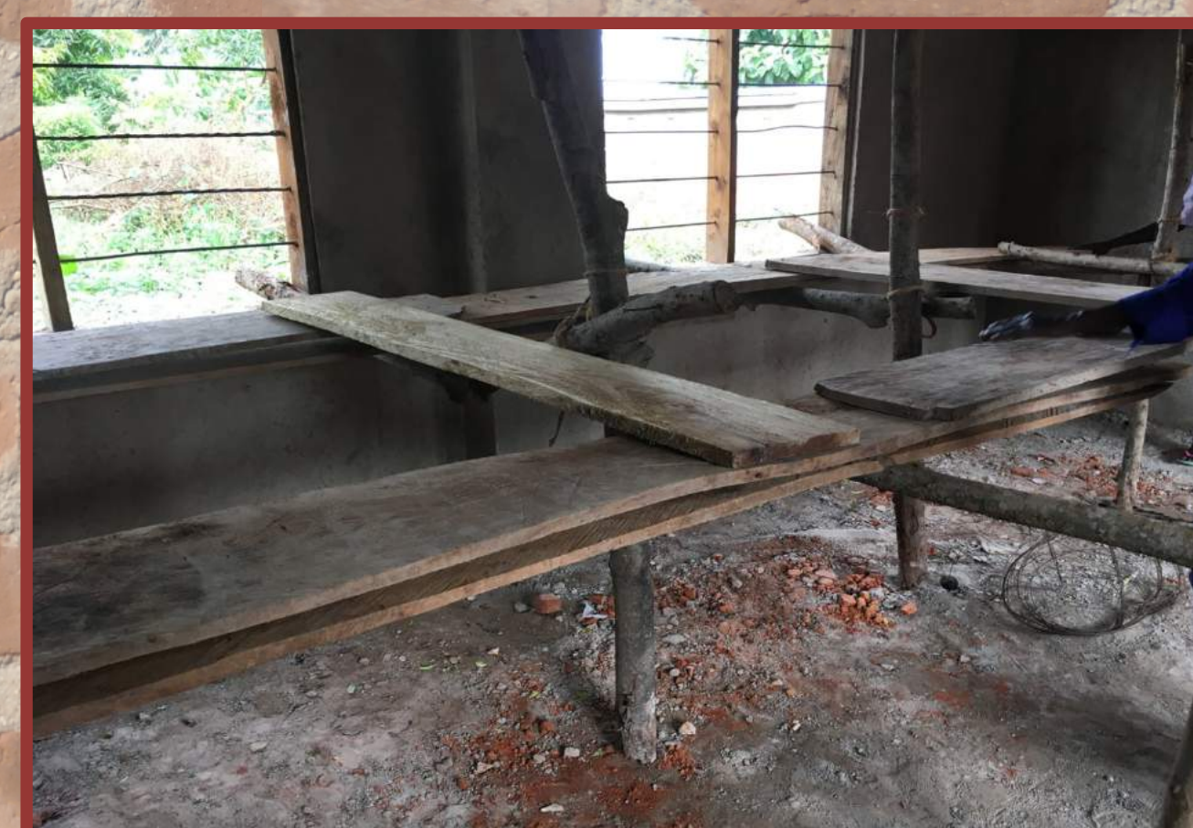
Image 3: Residual construction Material
